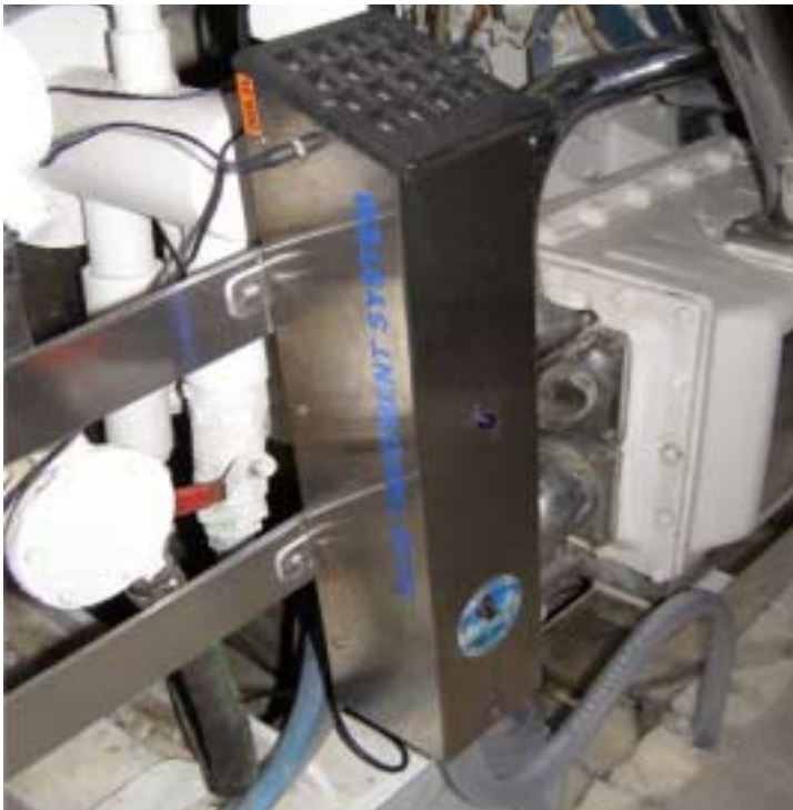
Holding Tank Ventilation System
